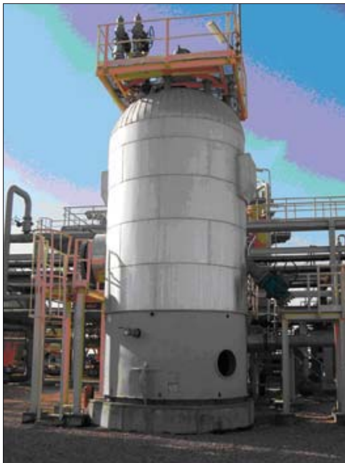
The mercury-removal unit at the Salam gas plant is loaded with 19 tons of a catalyst that consists of a high porosity, spherical mixed-sulfide adsorbent of different diameters (Fig. 2)
