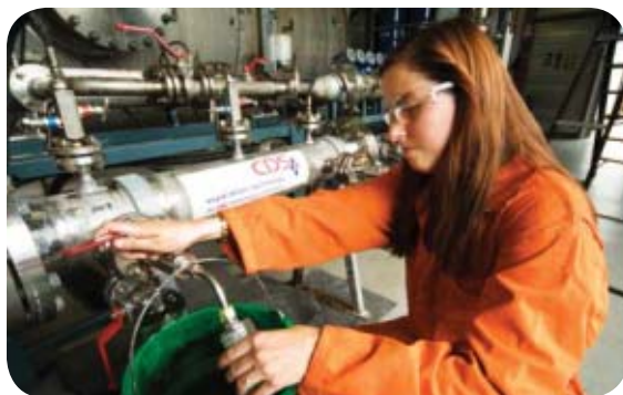
FMC Technologies' inline separation technology provides the company with a competitive advantage in subsea processing capabilities for deepwater development.
