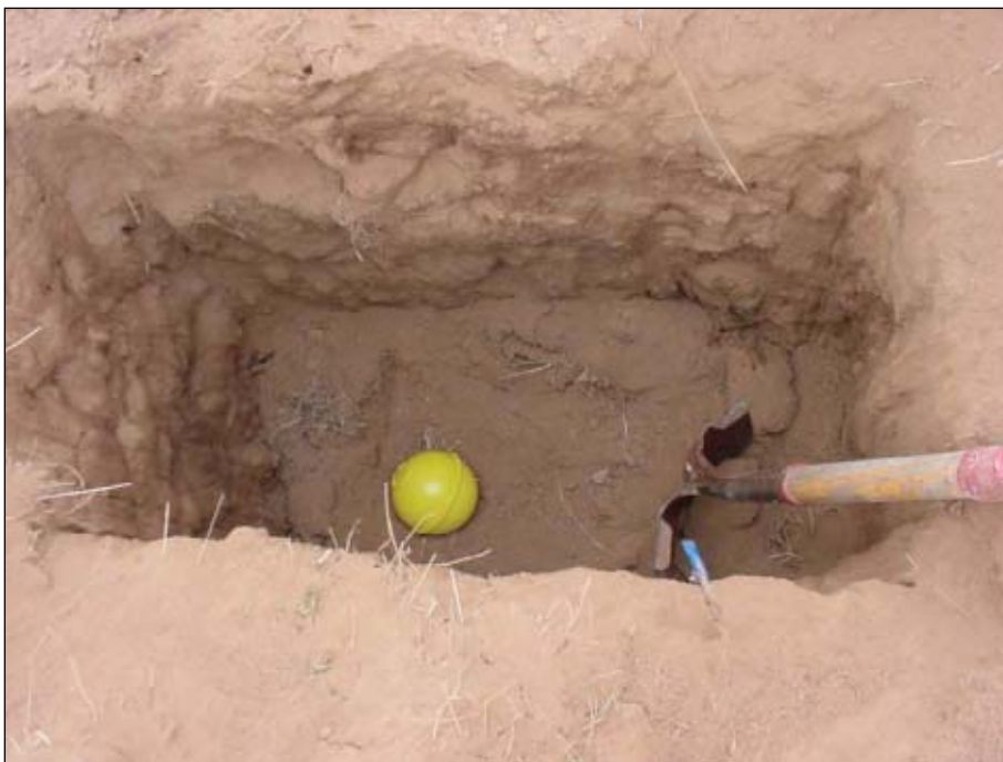
Backfilling the exposed pipes to a measured level allows placement of the ball marker at a known distance from the pipe (Fig. 4).
