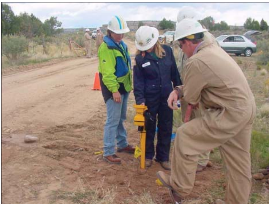
Marker read-write units load the ball location relative to the pipe, ID number, GPS coordinates, and any other identifying information onto the ball before burial. The same units will later use this information to confirm the precise location and depth of each marked crossing (Fig. 5).
