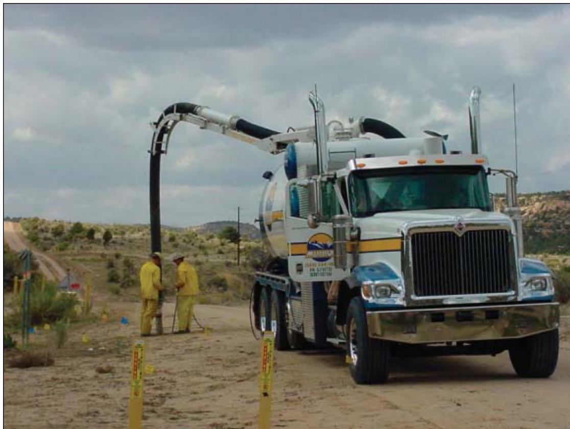
BP excavated each rural road crossing in its New Mexico region to expose buried pipeline (Fig. 2).
